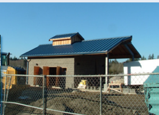
Kaiser Road Pump Station
