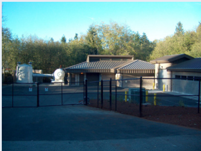
Martin Way Pump Station
