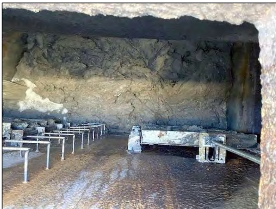
Pulpy mass in Budd Inlet Treatment Plant headworks
