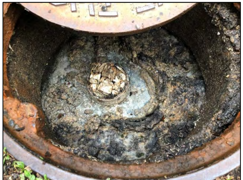
Styrofoam chunks in Empire Packing's grease interceptor
