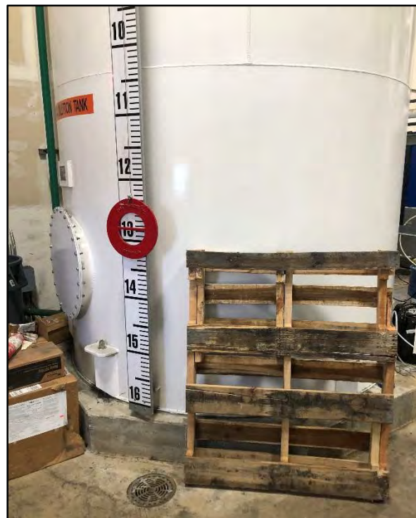
Ammonia diffusion tank and floor drain
