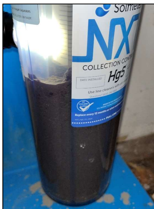
Non-compliant amalgam separator
