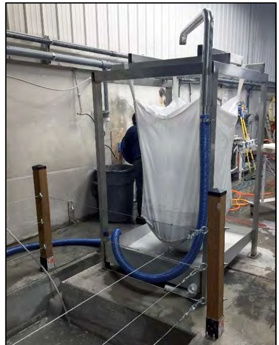
Bag filter for stone cutting wastewater
