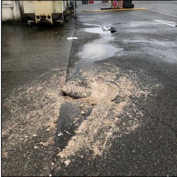
Grease interceptor overflow on March 13, 2023
