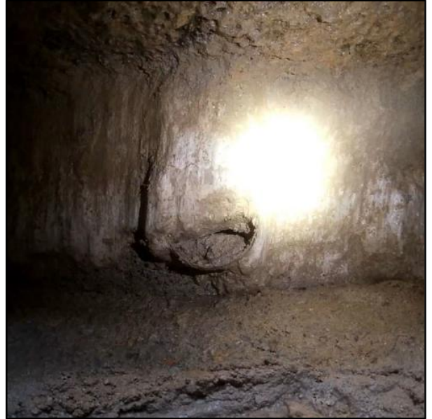
Blocked pipe between first and second chamber
