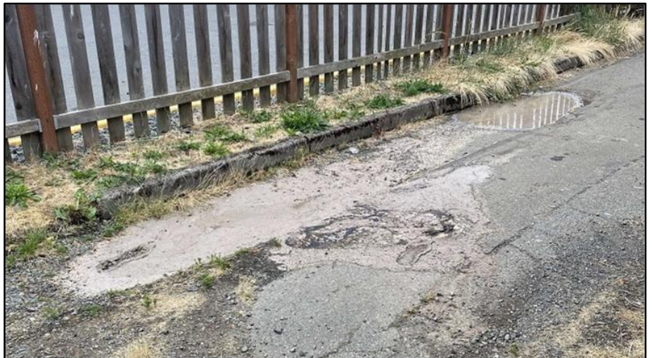
Sewage overflow in alley
