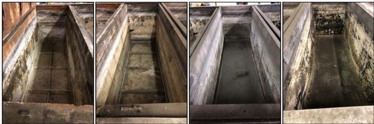
Empty Phosphatizing Tanks
