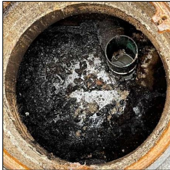
Port Taco Truck and Cantina Grease interceptor second chamber.
