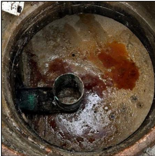
Port Taco Truck and Cantina Grease interceptor first chamber.
