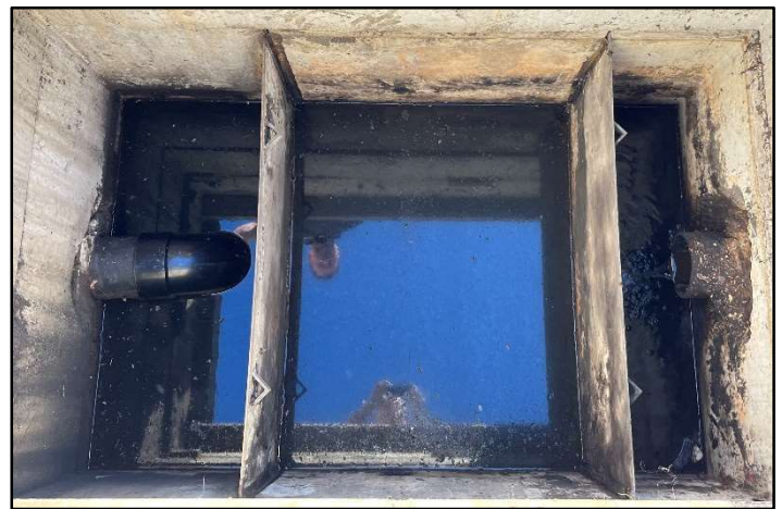
Oil and Water Separator after it was cleaned
