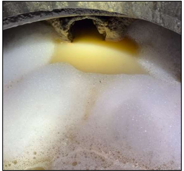
Outlet missing a pipe that prevents FOG from entering the sewer
