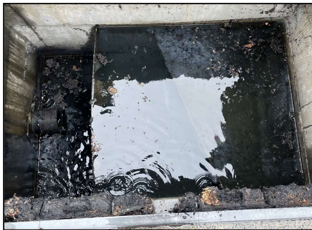
Oil and Water Separator overflowing due to excess sediment
