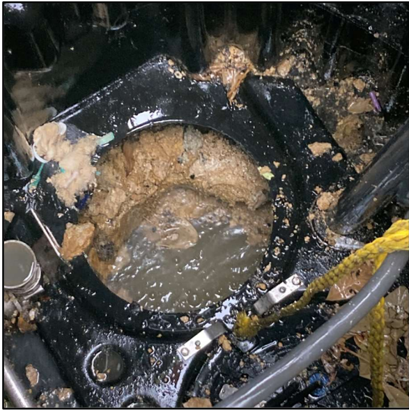
Grinder pump overwhelmed with FOG
