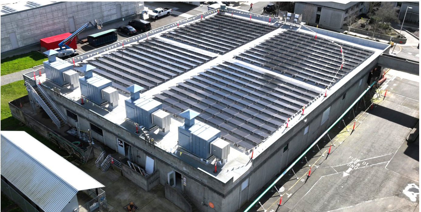
A solar array was installed as part of the Centrate Building Rehabilitation to further energy gains.
