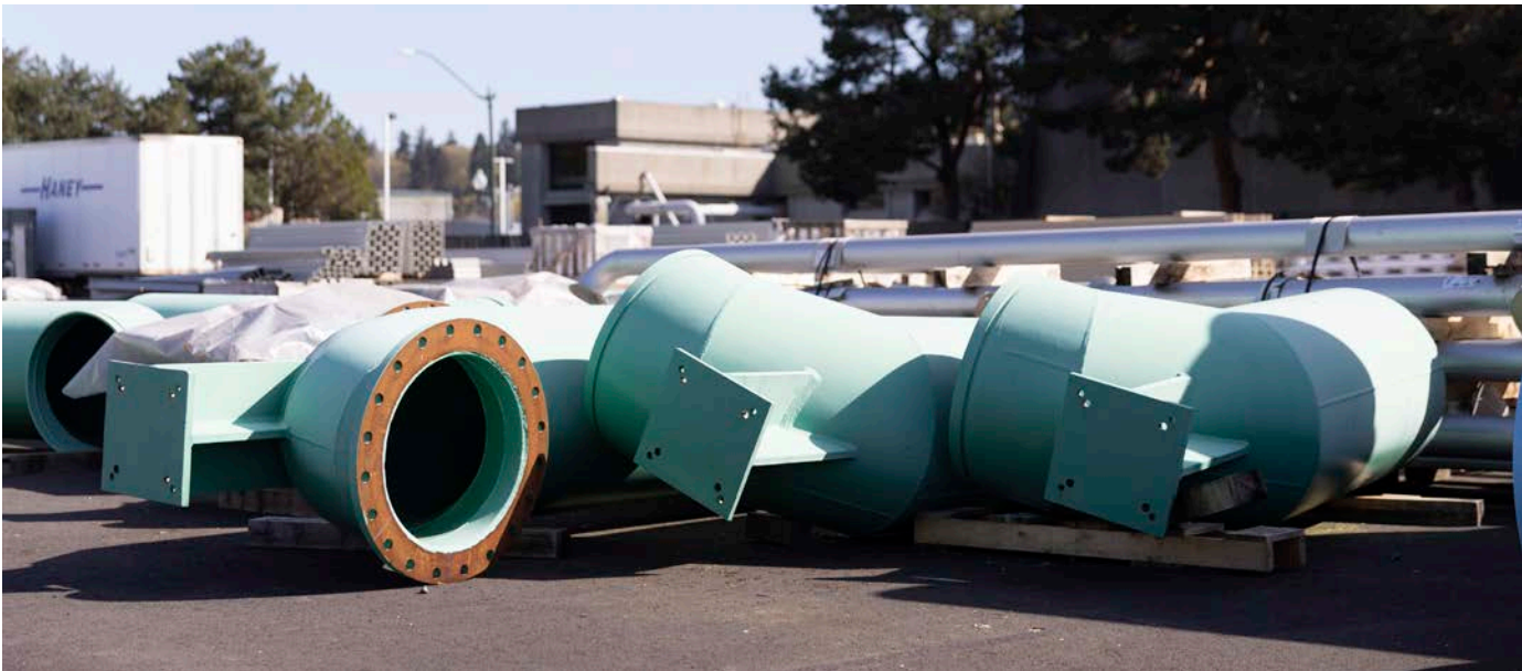
LOTT is continuously planning for new system capacity, to be built “just in time” to ensure future demands are met and to use the newest technology available.
